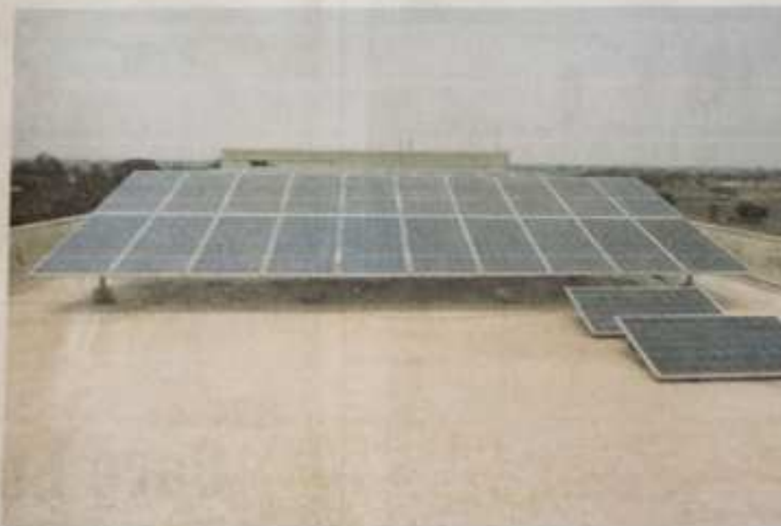
Fig.19. Solar PV System
