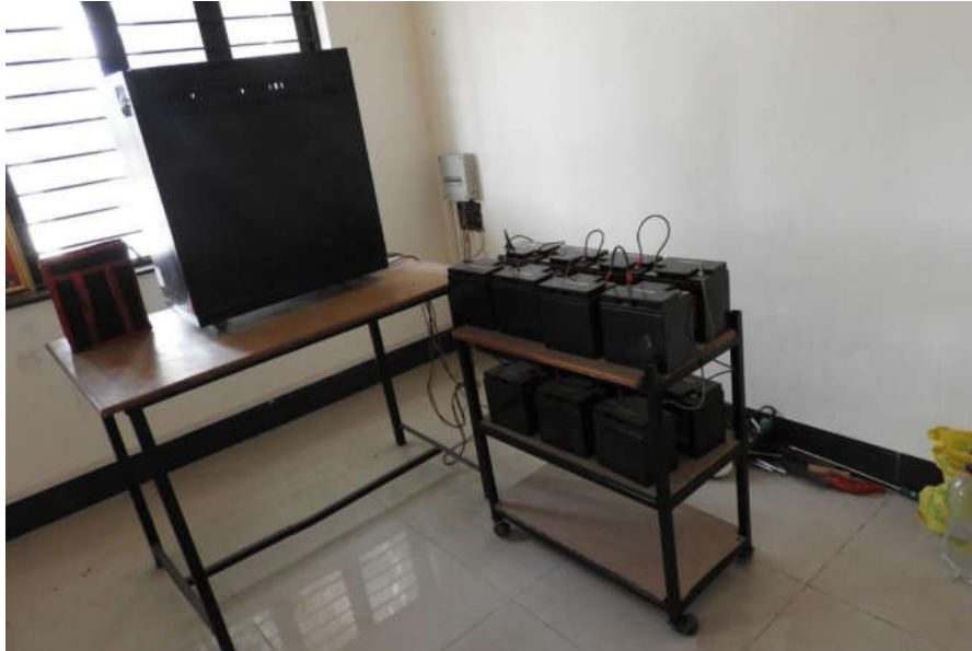
Battery Room with Exhaust Facility
