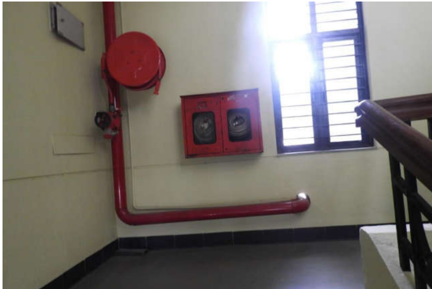
Fire Safety System
