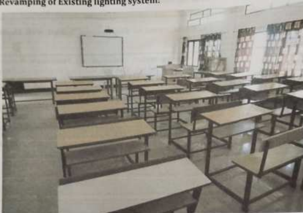
Fig. 4. : Existing Lighting System
